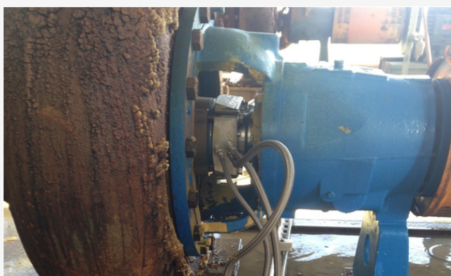
Slurry pump | Ethanol plant
